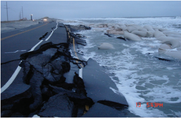
Storm damage at 'S' Curves portion of NC12. Source: NCDOT
